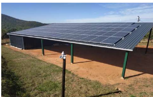
FIGURE 9: Sigcineni 35 kWh Solar PV Mini-grid with 200 kWh Battery Storage
