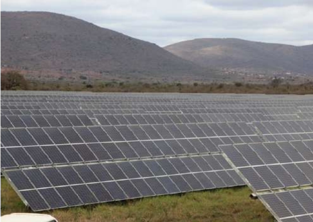
FIGURE 3: Lavumisa 10 MW Solar Plant Owned and Operated by EEC
